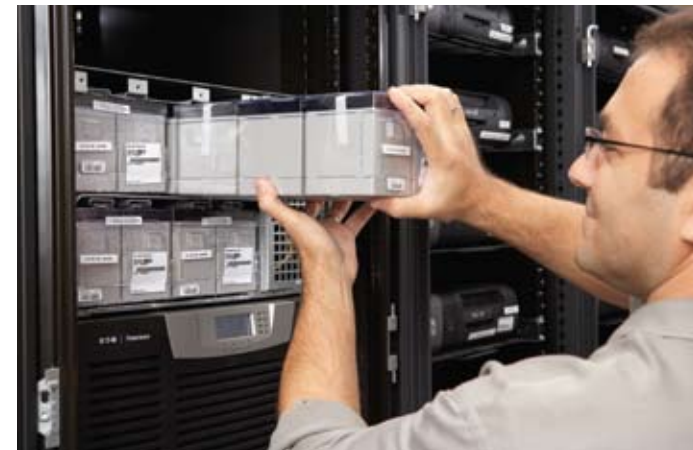
IT staff can easily replace battery modules.
