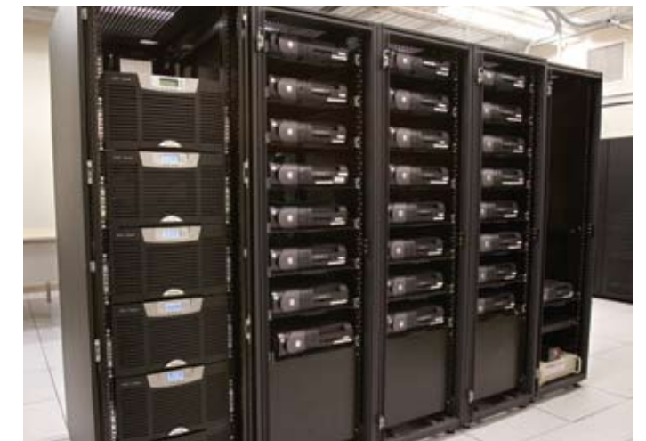
The BladeUPS remains cool even in a data center full of servers.
